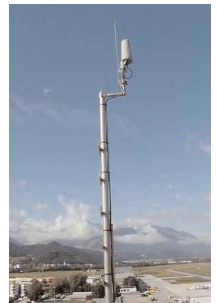
One of the nine Remote Unit Antennas of the Innsbruck Wide Area Multilateration System
